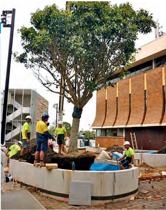
A HEAVY lift crane was used for landscaping at Hutchies' Queensland Emergency Operations Centre at Kedron which involved transplantation of three Moreton Bay figs into planter boxes.
