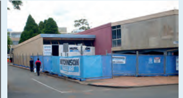
Toowoomba's Regional Council building is being refurbished to include a new Customer Service Centre.
